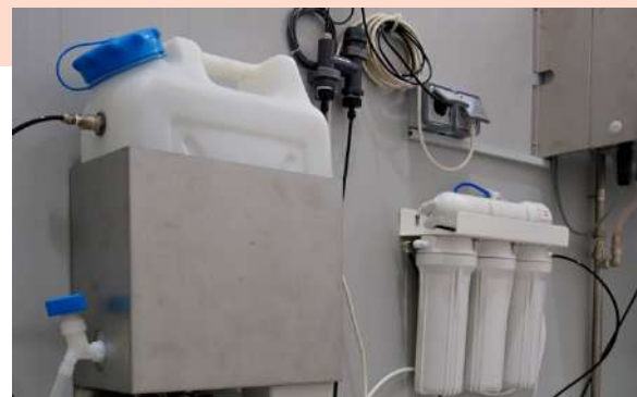
Water Treatment systems
