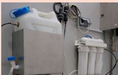
Water Treatment systems
