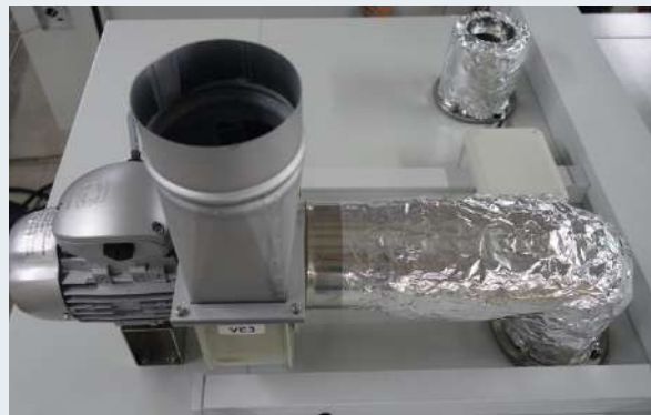
FLUSHING / PRESSURE RELIEF SAFETY
